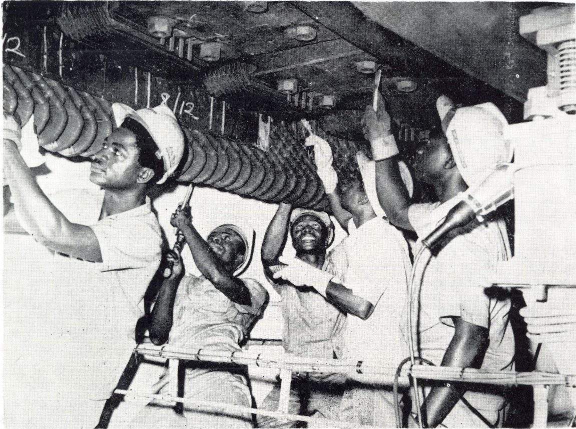
Technicians busy at repair work on one of the turbines at Akosombo Power House
